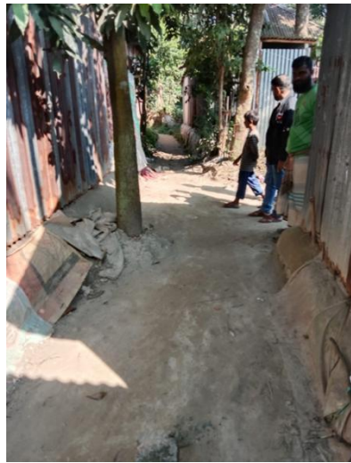
Figure IV.1: Existing Situation of Footpath at Mouzzakanda LIN
