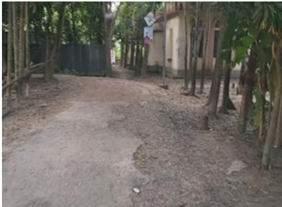
BOAL-R-06: Improvement of Road by DBC Starting from near Boalmari George Academy to Amgram Chalinagor Road via Govt. College Ch. 0.00-1416.00m. At Ward No-05, Under Boalmari Pourashava, Faridpur. (Total Length=1416.00m).
