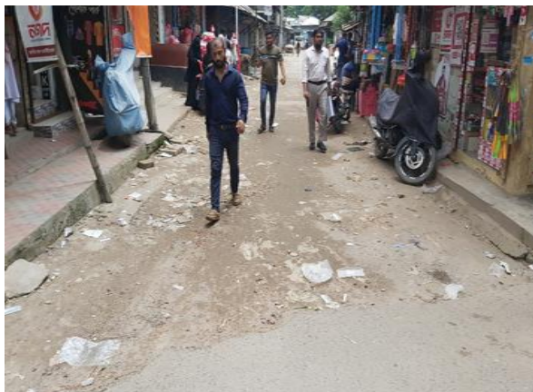
BOAL-R-19: Improvement of road by DBC Starting from the front side of Sobhan Market to Bangabandhu road via Boalmari Jame Mosque Ch. 0.00-90.00m. at Ward no.-03, Under Boalmari Paurashava, Faridpur. (Total Length=90m).
