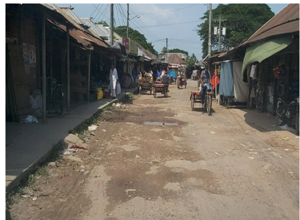
BOAL-R-17: Improvement of Road by DBC at Gunboha Starting from West Boundary to East Boundary via Puraton Bridge of Paurashava near Darul Ulum Hafejia Madrasah via Anderchota Bridge Ch. 0.00-1780.00m. Including 02 Nos RCC Pipe Culvert at (Ch. 670.00m & 850.00m), Installation of Street Light 61 Nos. at Ward no.-01 Under Boalmari Paurashava, Faridpur. (Total Length=1780.00m).
