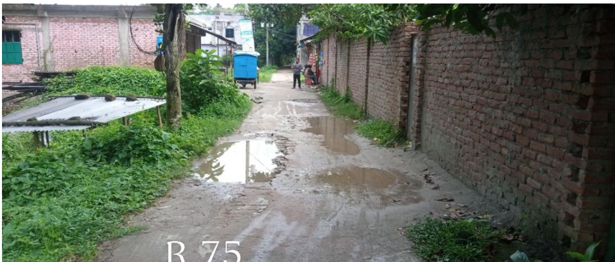
R-075:Construction of Road from Cumilla- Chadpur Road to Rail Line (Ch. 0+00 to 0+829m) including Protection Work at (Ch. 0+200 to 0+390m, L/S), (Ch. 0+263 to +297m, R/S), (Ch. 0+308 to 0+363m, R/S), (Ch. 0+522 to 0+561m, R/S) & Installation of 28 Nos. Street Light in Ward no. – 03 under Haziganj Paurashava, Chandpur.
