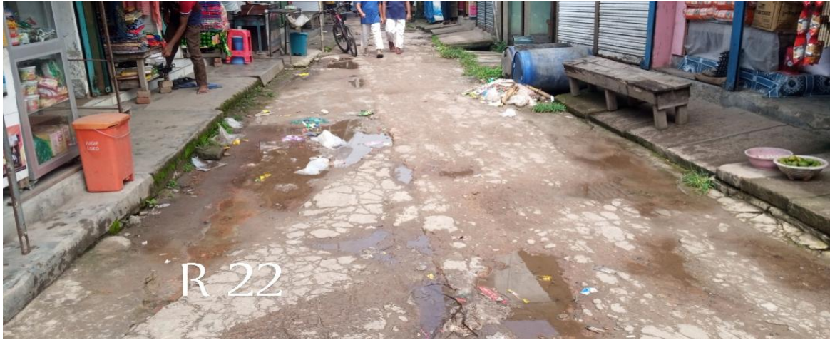
R-022:Construction of Road from Cumilla- Chadpur Highway to Sharda Ferry Ghat Road (Ch. 0+00 to 0+134m) & link Road Starting from Mojumder Cloth Store to Fish Bazar (Ch. 0+00 to 0+22m) Total Length= 156m & Installation of 06 Nos. Street Light in Ward no. - 02 Haziganj Paurashava, Chandpur
