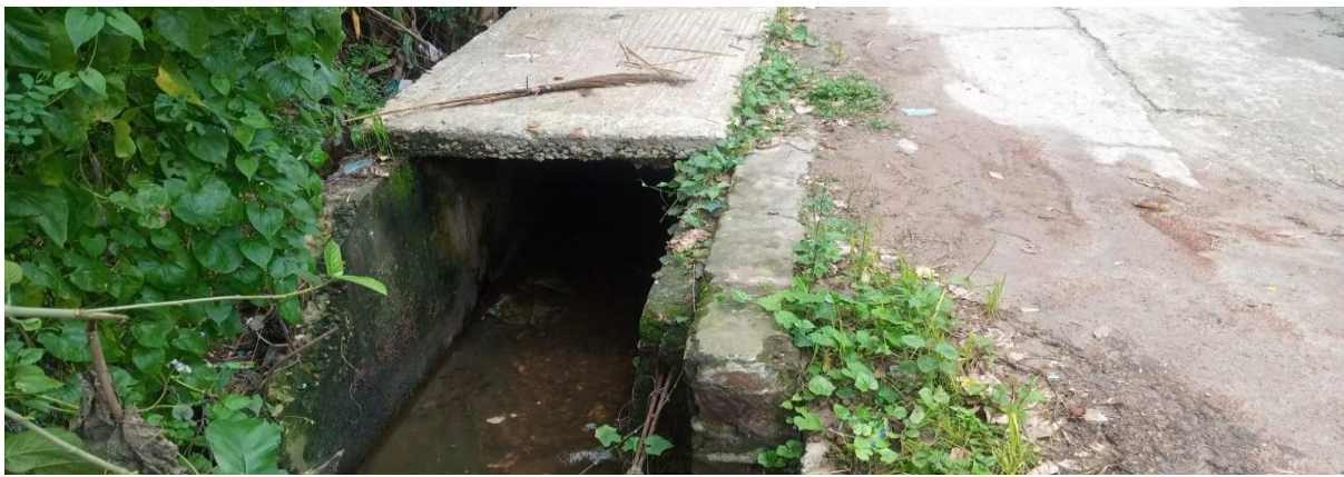
D-14:Construction of RCC Drain Starting from Beside Cumilla-Chadpur Road to Mithania Canal via Bilaway Hazi Bari Road (Ch. 0.00-860.00m) at Ward no-03, Haziganj Paurashava, Chandpur (Total Length=860.00m).
