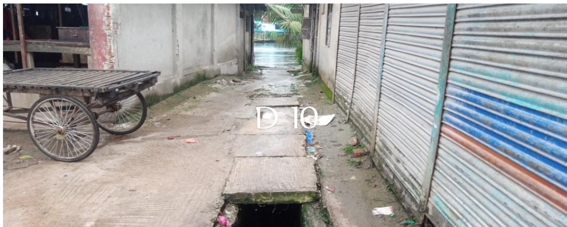
D-010: Construction of RCC Drain Starting from Haziganj Bazar Hawkers Market to South direction Dakatiya Canal (Ch. 0.00-275.00m) at Ward no-05, Haziganj Paurashava, Chandpur (Total Length=275.00m).
