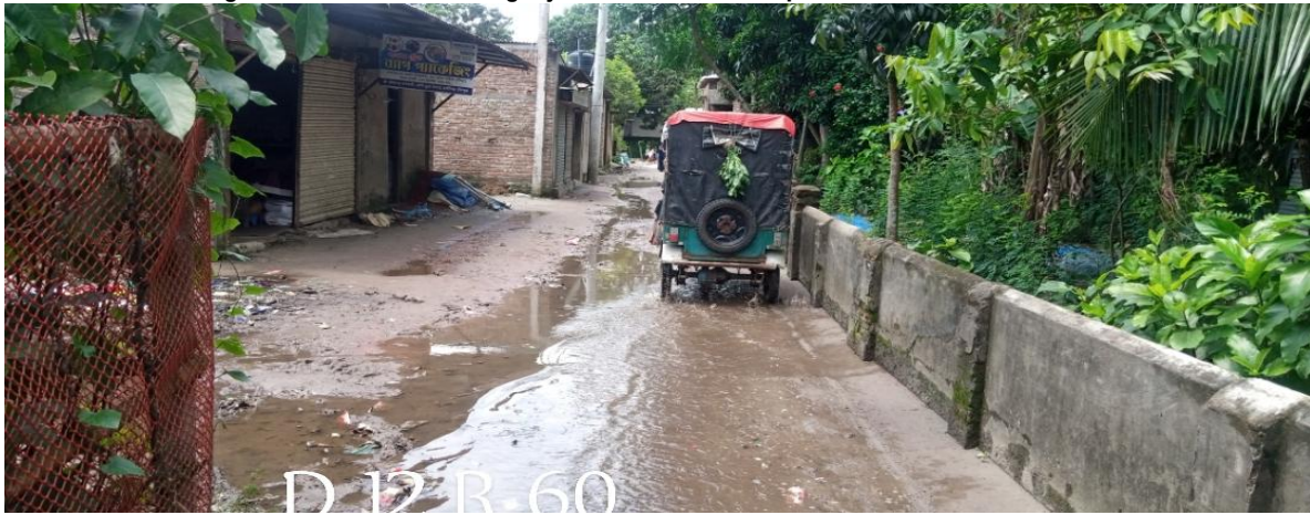
R-60:Construction of Road from Taragor Md Siraj Uddin to Talukder House (Ch. 0+00 to +0689m) & Link-02 (Ch. 0+00 to +070m) & Link-03 (Ch. 0+00 to 0+091m) Total Length= 850m & Installation of 31 Nos. Street Light in Ward no. - 08 Haziganj Paurashava, Chandpur.
