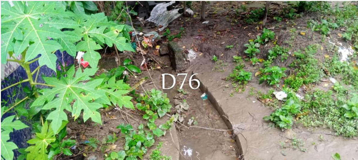
R-76: Construction of RCC Drain Starting from Radhunimora Mazar to North Direction Degree College (Ch. 0.00-263.00m) at Ward no-11, under Haziganj Paurashava, Chandpur. (Total Length=263.00m)
