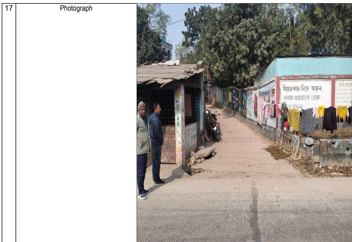
D-157: Construction RCC Drain Starting from Nungola KDC gate to Asraful house (Ch: 0.000-188.00m) & Link drain (Ch: 0.00-376.00m) Total Length= 558.00 m in Ward No. 06 under Rohanpur Pouroshova, Chapainawabganj.
