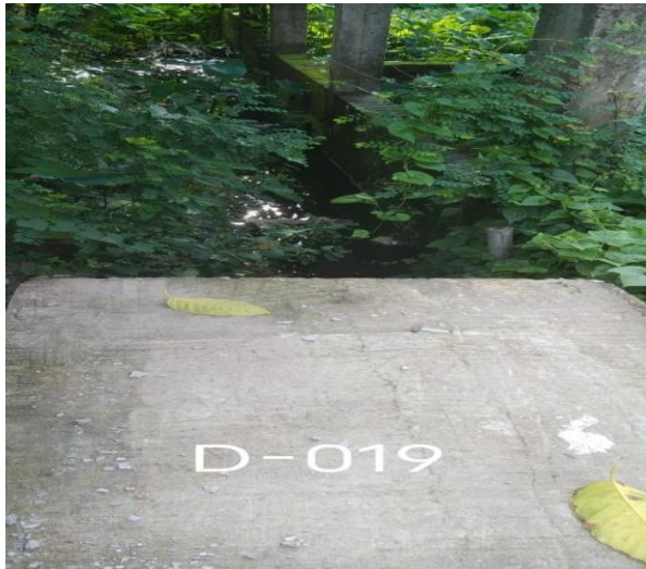
Photo , Haziganj- Drain -19
