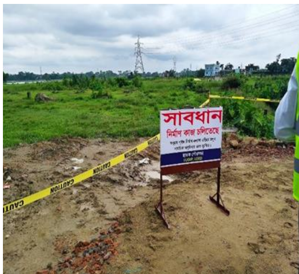
Safety sign in Chhatak pourashava site
